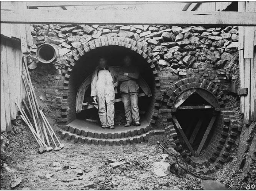
17.1 Men standing in opening of unfinished sewer in the 1880s. Image, Edgar Sutton Dorr Photograph Collection, Boston Public Library.
